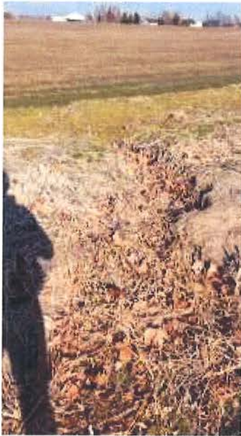
Photo 1. Drainage Erosion Rills
