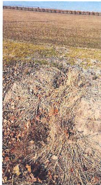
Photo 2. Drainage Erosion Rills
