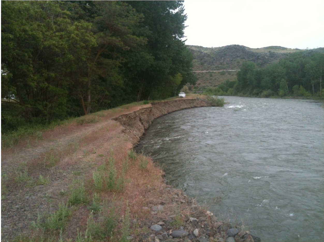
Figure 5 - May 2012 Ramblers' Park levee undercut and collapse at 2 year flow, the year after 2011 approximately 15 year peak flow. In foreground in 1996 failure, car in background is parked just upstream from 2006 failure.
